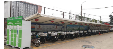
Street charging station
